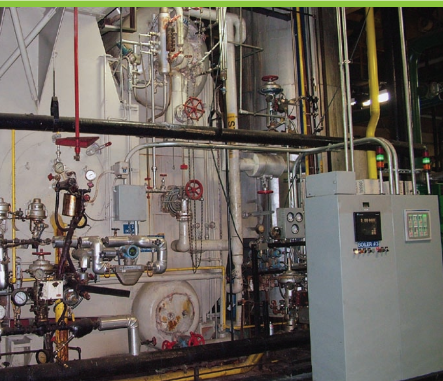
The steam system at Goodyear's Union City plant is served by four dual fueled (natural gas and No. 6 fuel oil) boilers, such as the 60,000 lbs/hr boiler pictured above.
