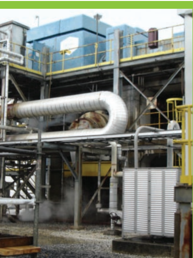
Increasing condensate recovery could save nearly 88,000 MMBtu per year.
