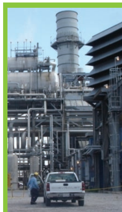
The east heat recovery unit at Dow's St. Charles Operations in Hahnville, Louisiana.
